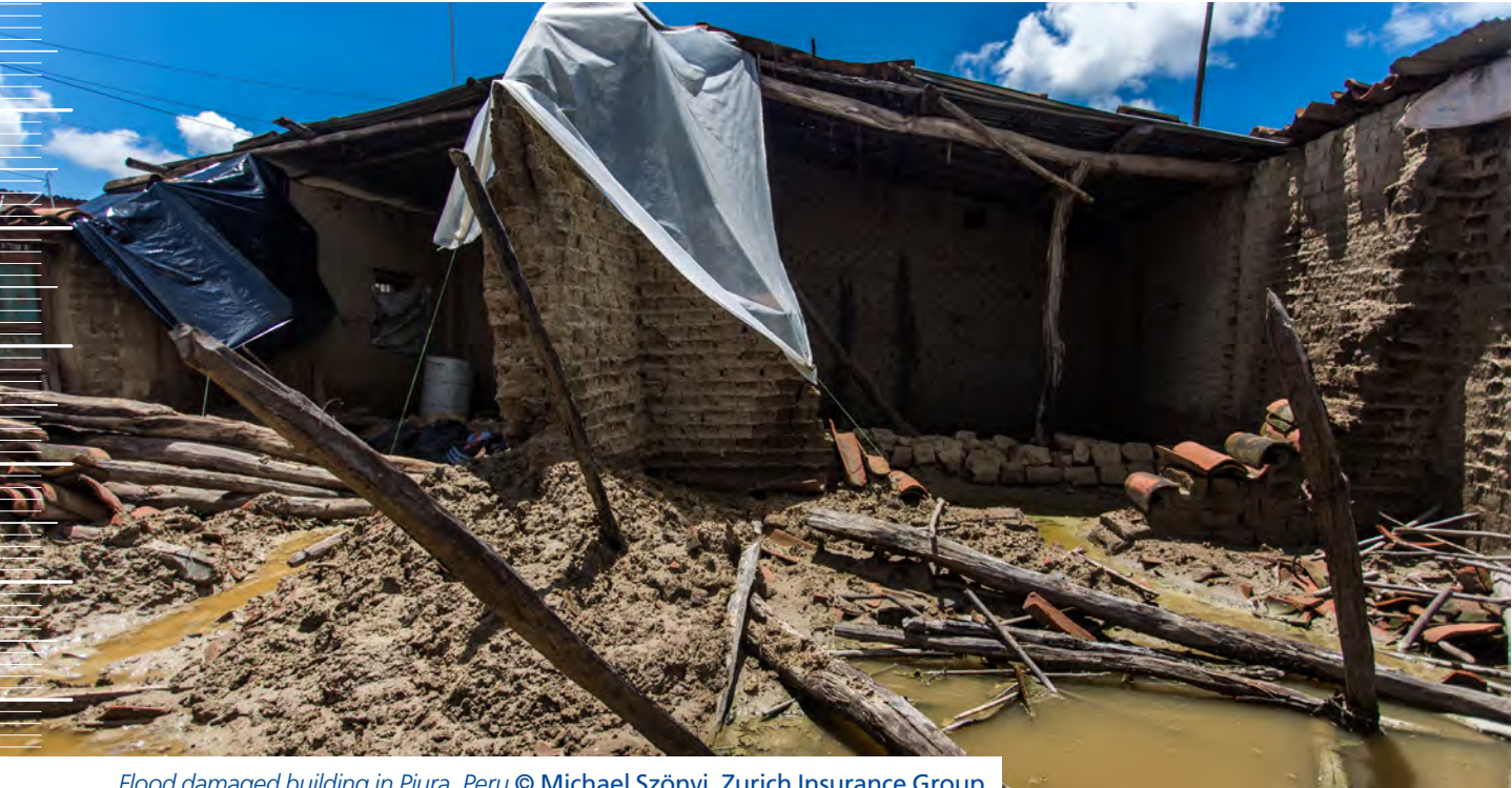
Flood damaged building in Piura, Peru © Michael Szönyi, Zurich Insurance Group
